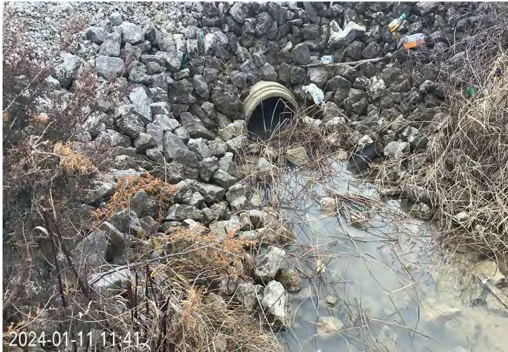
Photograph Location 4. Representative view of an existing culvert within the Project area. Photograph taken facing south.
